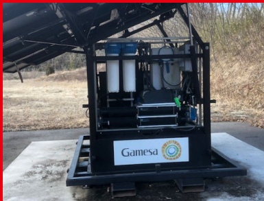
Solar-powered water purification equipment
