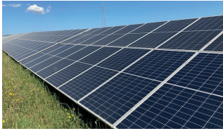
Socovos power plant in Spain
